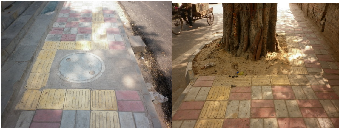
Photo 2.2 Incorrect tactile pavers layout on footpaths.
